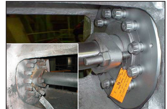
Failed valve with leak seal injection port and 5-ring set installed.
